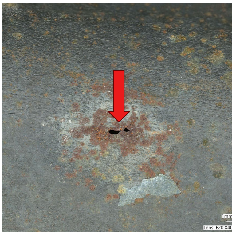
Figure 20: Evidence #3 - pipe interior surface in area of the leak.
