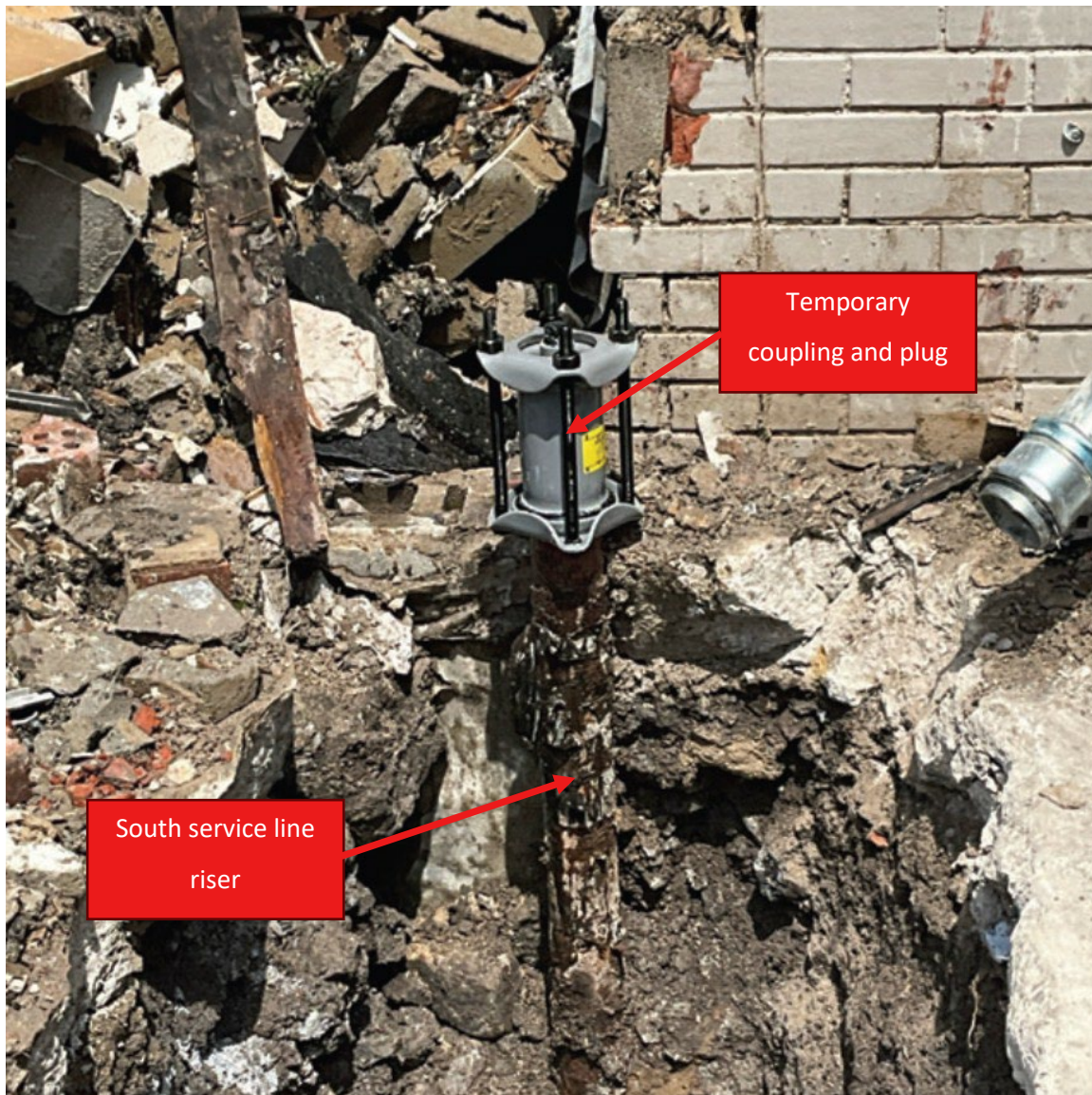
Figure 8: Pressure drop test #2, on June 24, 2025, at south service line, against coupling and plug on vertical riser, outside of building.
