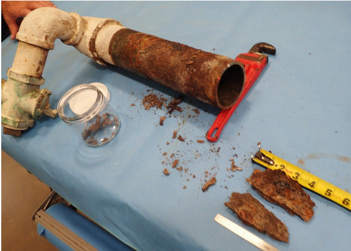
Figure 18: Evidence #3 with corrosion buildup removed.
