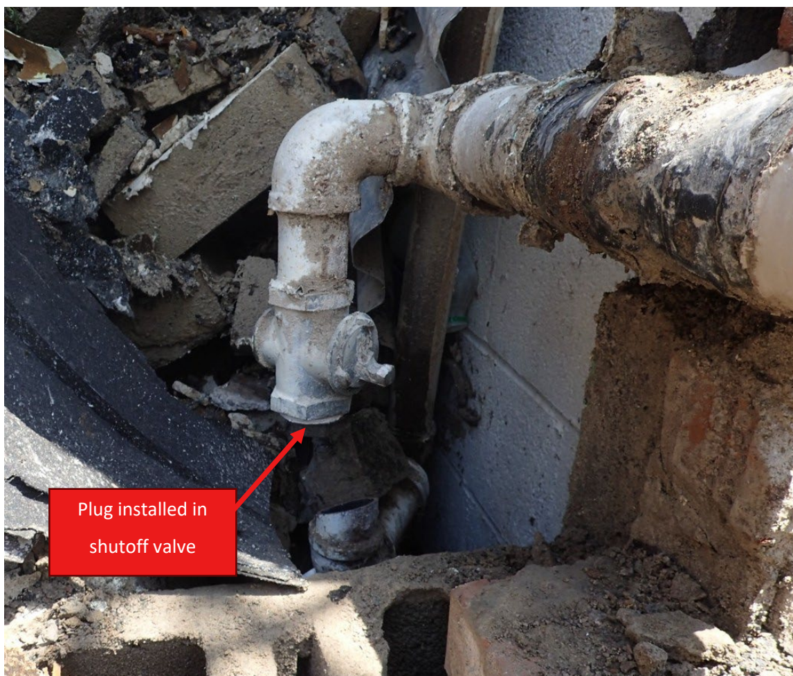
Figure 7: Pressure drop test #1, on June 24, 2025, at south service line, against plug on downstream side of shutoff valve.
