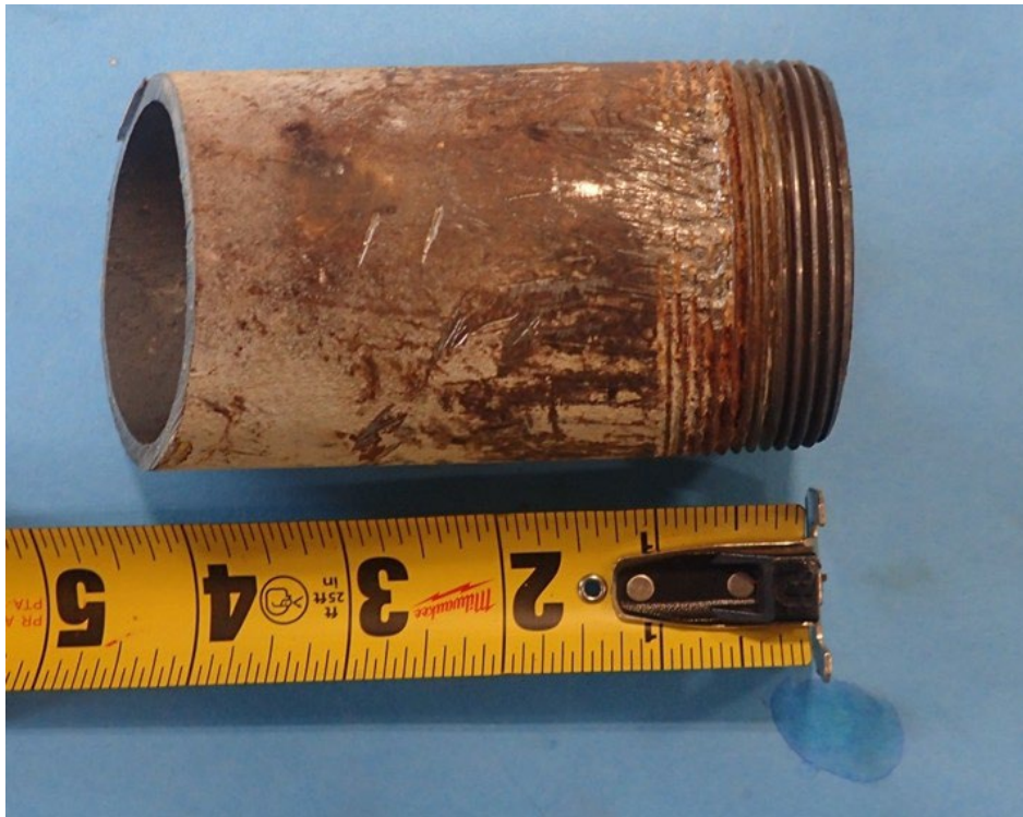
Figure 12: Evidence #1 - south service line, pipe nipple downstream of valve just inside wall.
